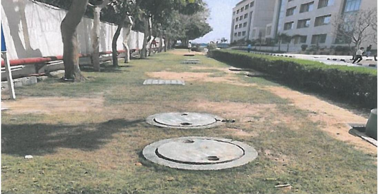
Recharge pits & Tanks at J. S. University
