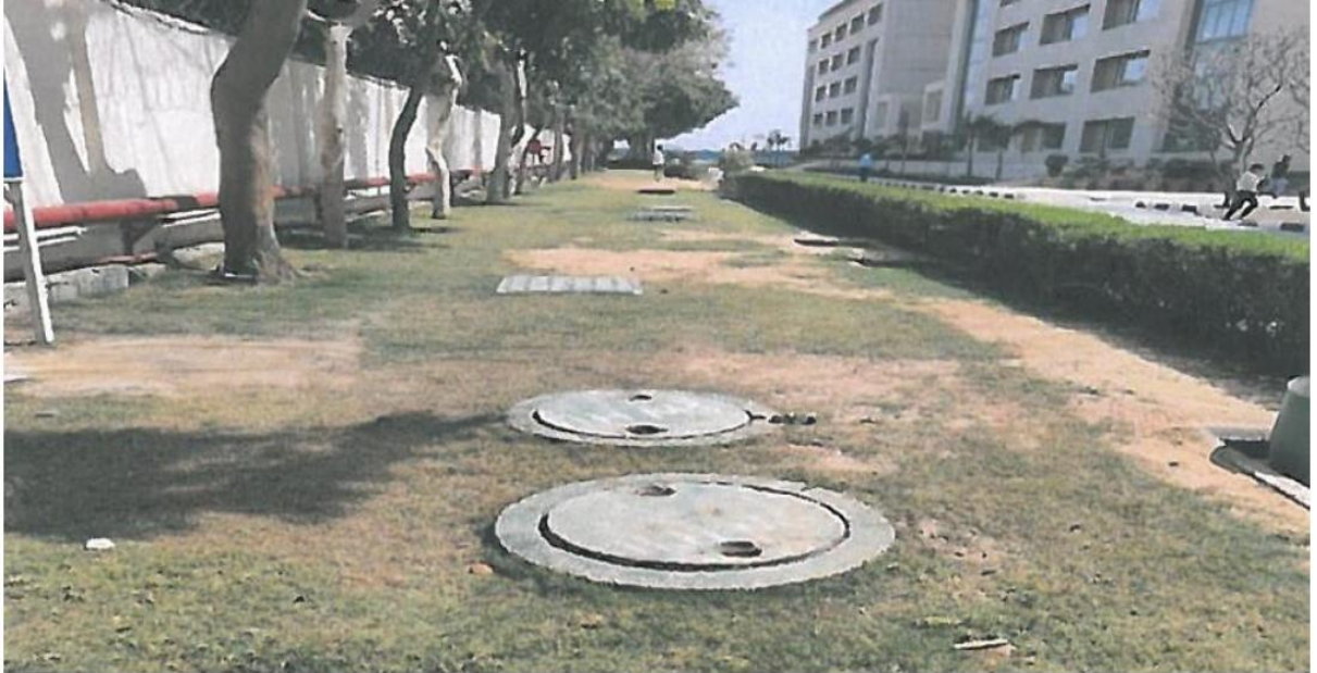
Recharge pits & Tanks at J. S. University
