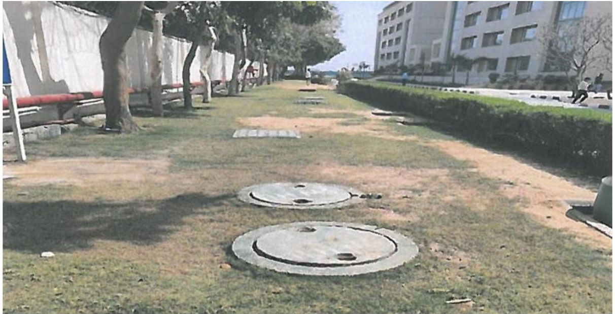
Recharge pits & Tanks at J. S. University
