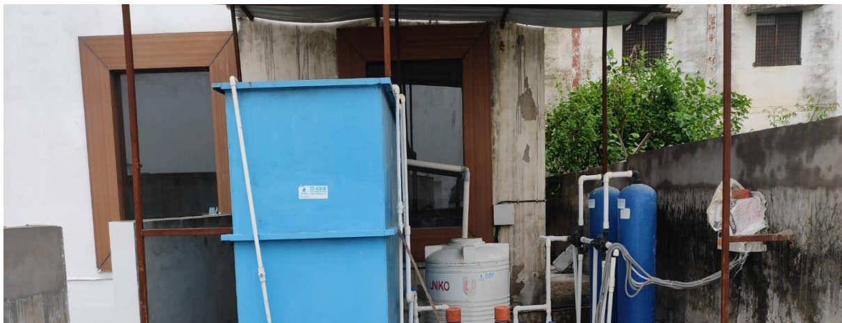
Sewage Treatment Plant
